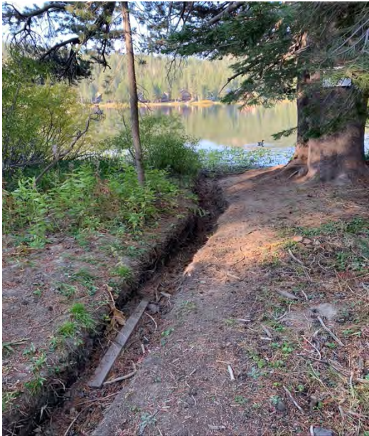
Unauthorized Drainage Improvement at the end of Dulzura Road
